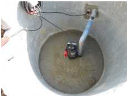
Station de relevage
