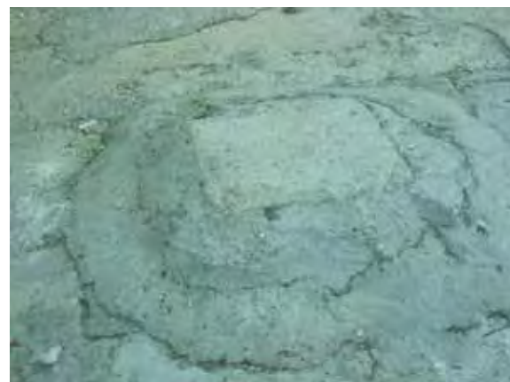
Photo 9.4 Drains covered improperly.
