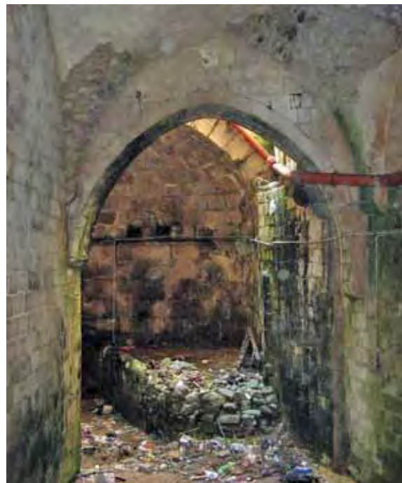
Photo 9.2 Bare pipes of the sewage network.
