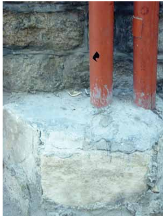
Photo 9.1 Worn out pipes of the sewage network.
